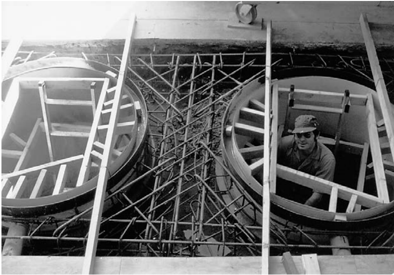
Figure 20-33. Mark Connaughton in the process of constructing underground silos in Southern California for CryoSpan.
