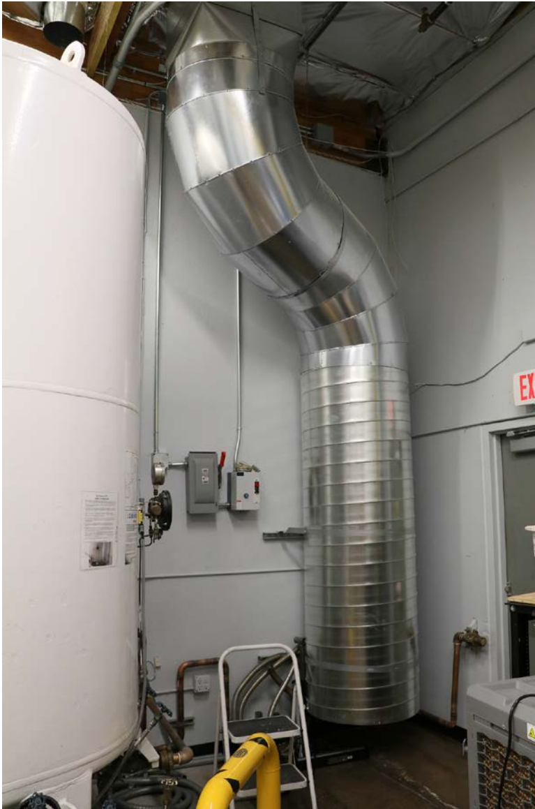
Figure 20-32. One of several large ventilation ducts in Alcor's patient care bay. Fans on the roof are activated automatically if an oxygen sensor suggests a buildup of nitrogen in the air.
