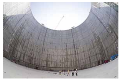
A view of the sky from about 60 meters underground; the tank will have a storage capacity of 250,000 kiloliters, an inner diameter of 72.0 meters, and a depth of 61.7 meters (photo taken in Summer 2010).
