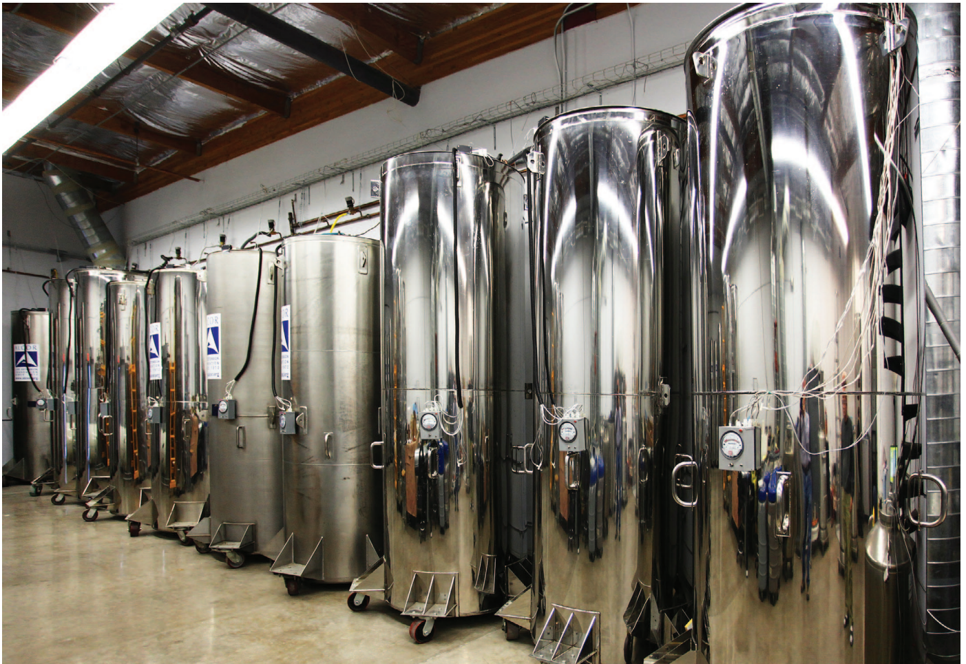
The Alcor Patient Care Bay. All dewars are equipped with level detectors and alarm systems. The lines above the dewar allow for automated dewar refills from a larger bulk tank.
